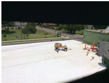
... and (nearly) after. No more leaks!
